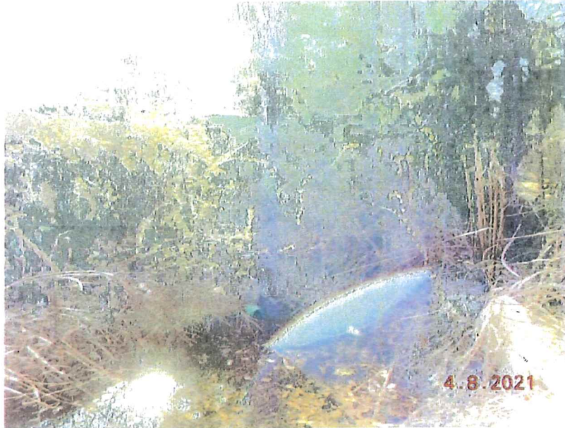
Photo 3 – View from 217 Cocasset of excavated area looking towards 227 Cocasset. Note height of fill placed on 227 Cocasset.
