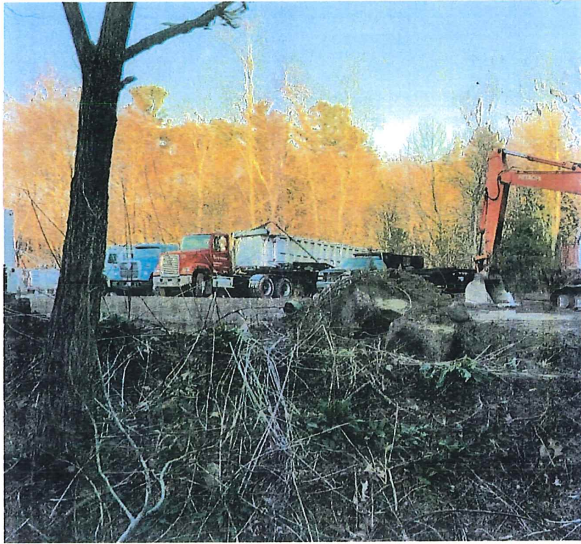
Photo 4 – View looking northeast from 217 (left side of photo) towards 227 Cocasset Street. Note 4-inch PVC pipe at middle center along with soil and boulders that had been removed from 217 Cocasset Street.
