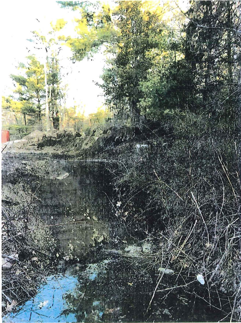
Photo 2 – View of Excavated area on 217 Cocasset taken 4-8-2021 showing removal of 4-inch PVC pipe by owner of 227 Cocasset Street.
