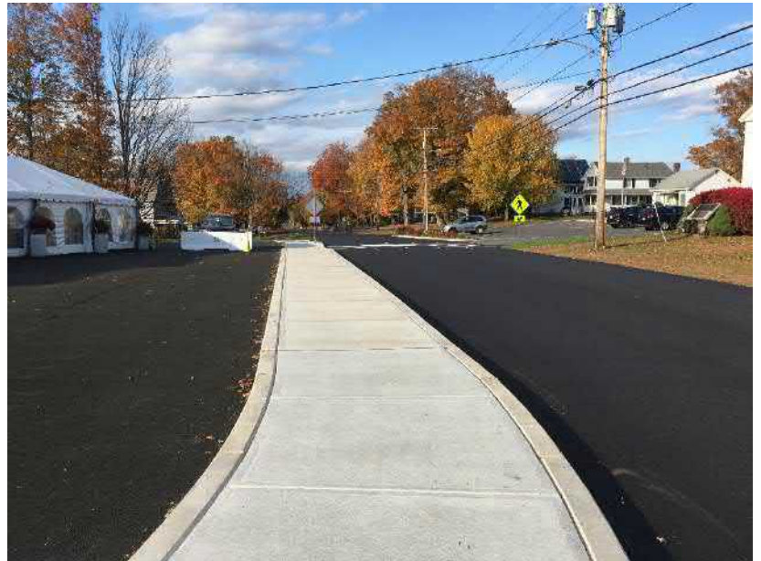
AFTER: The well defined parking area in front of the Whately Inn provides space for both parking and a seasonal tent for outdoor dining.
