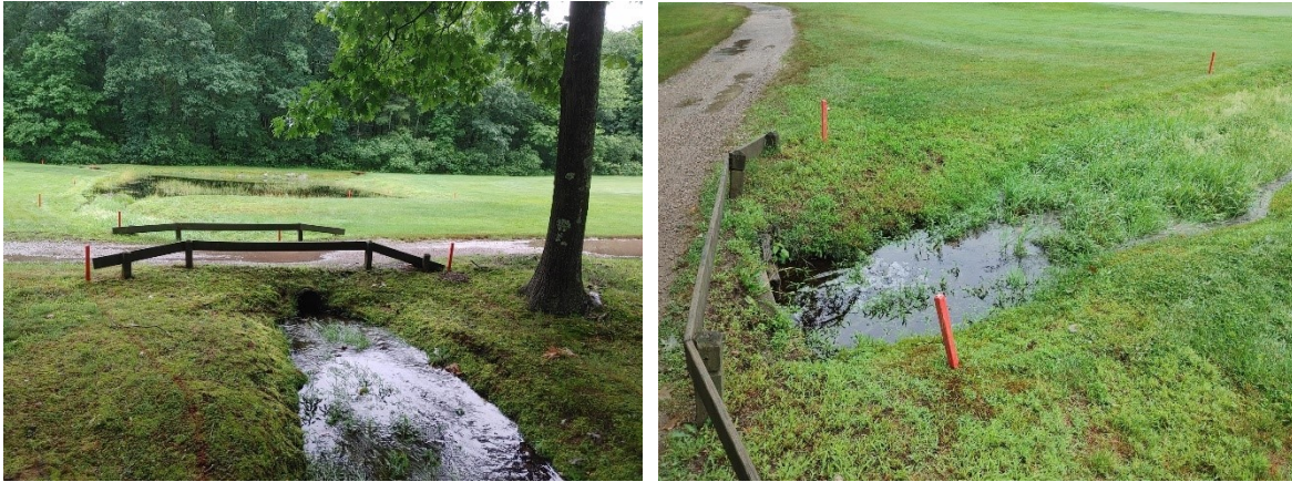
Left Photograph: View facing south of existing undersized culvert and subject pond.
