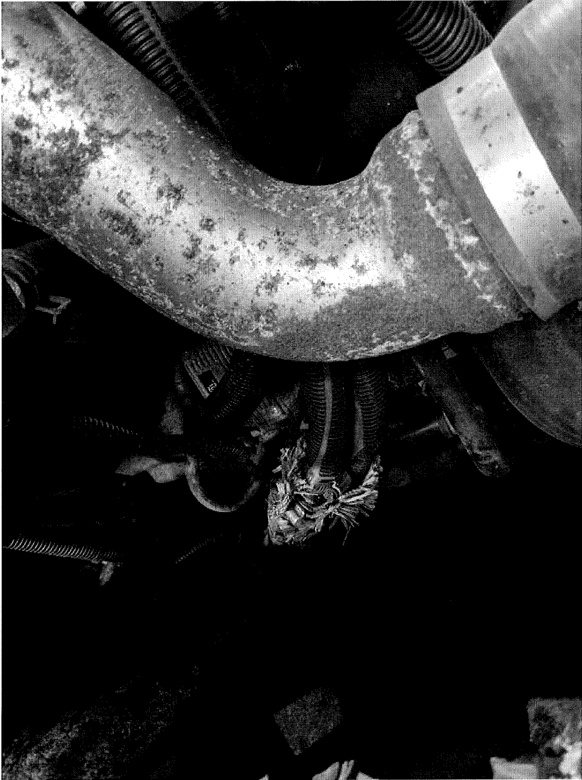
Figure 2- rotting air cooler line
