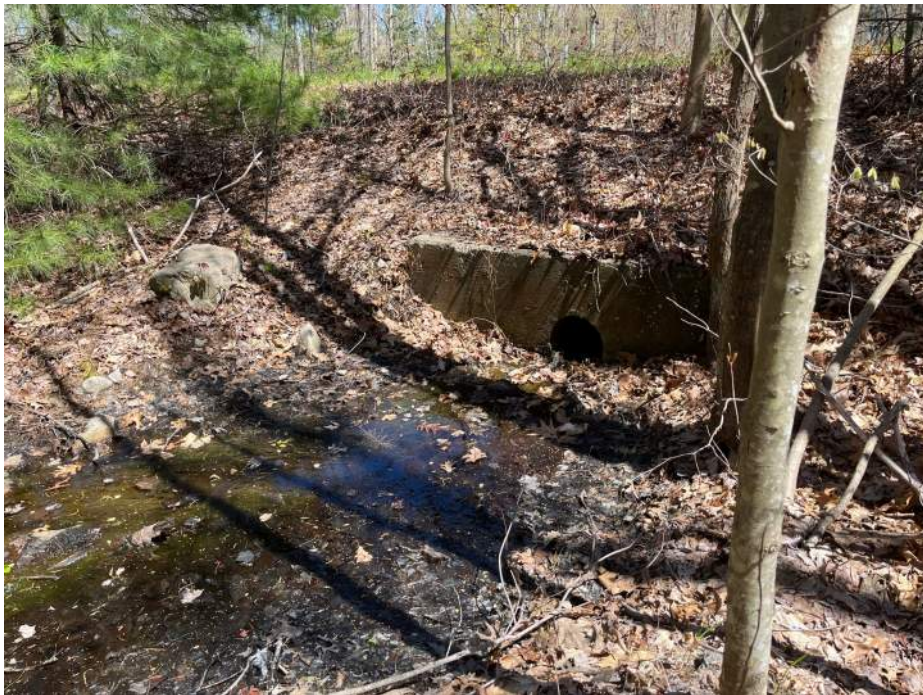
Photo 6: Culvert passing flow from C-series BVW into drainage pipe under Walnut Street.
